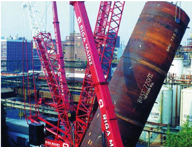
On-site manufacture of two waste acid tanks. Diameter 6.800 mms, height 27.400 mms, volume 900 m 3
